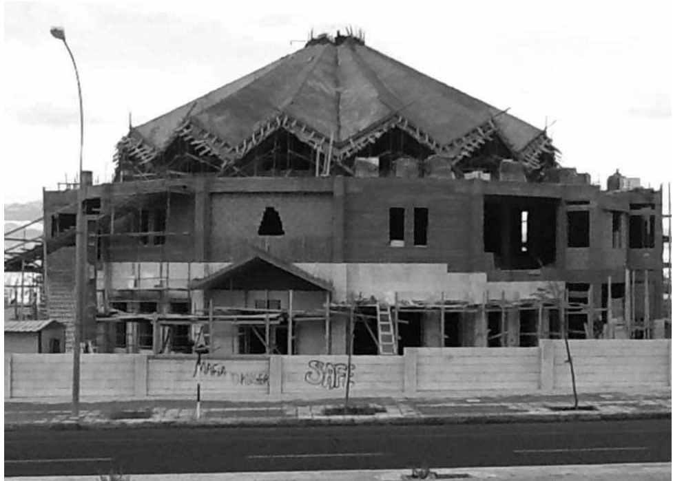
The construction work for the Church of Stella Maris in Aqaba as it was at the end of March.
